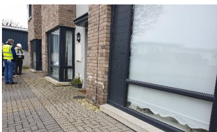
Figure 4 Moisture adsorption/passage-Level access, sills at ground level permeable paving-and considerable slope!!
