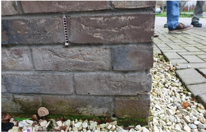
Figure 2 Moisture adsorption/passage to brickwork, drainage not doing its job to dispose surface water from the building- -French Drain-stone!!
