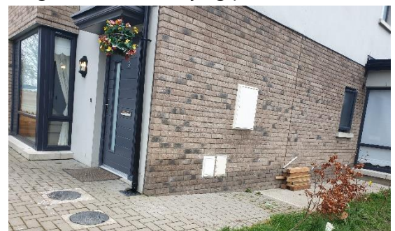
Figure 3 Moisture adsorption/passage-permeable paving not successful in disposing surface water from the building. Note also grass area!
